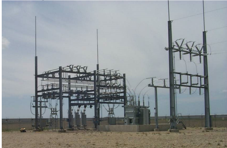
Figure A1 - 6: Distribution Substation
